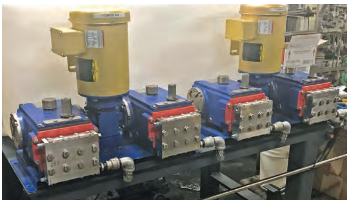
Chemical boiler feed at a power plant. Four MT8 pumps running off two gearboxes and two motors shows its duplexing capability.
